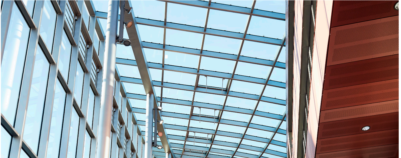
Glass roof of the library building of the University of Marburg, Germany.
